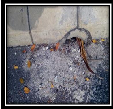
Figure 2: Scupper Drain clogged by new road paving
