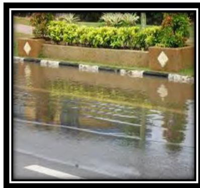
Figure 3: Stagnant water due to clogged drainage
