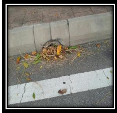
Figure 1: Scupper Drain clogged by leaves and rubbish
