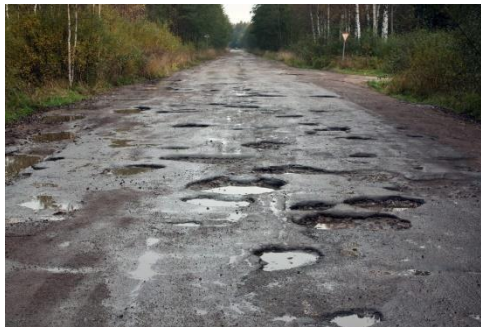
Rajah 2.9: lelubang pothole
