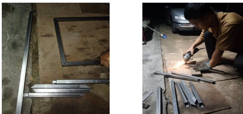
Figure 3.4 ii: MIG welding is used to join hollow iron& Grinder to cutting iron
