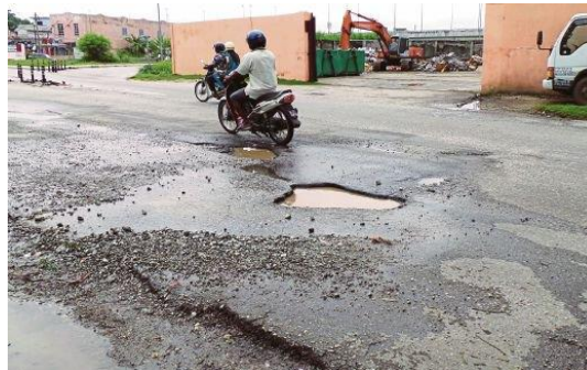
Figure 3.3.1.1: Pothole at Sentosa Klang
