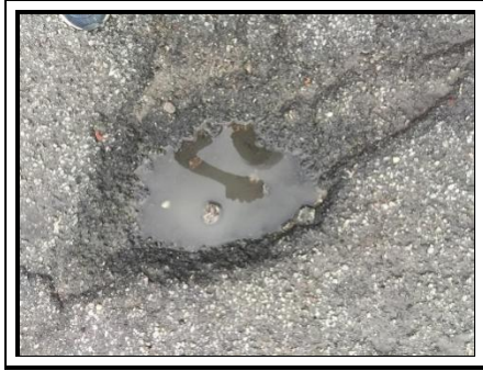
Figure 1.5: Pothole at gate B entrance
