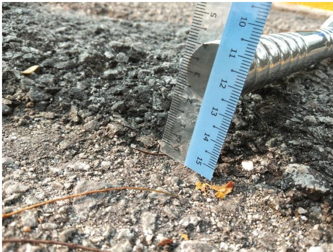
Figure 3.4.2.2: Measure the depth of pothole using ruler
